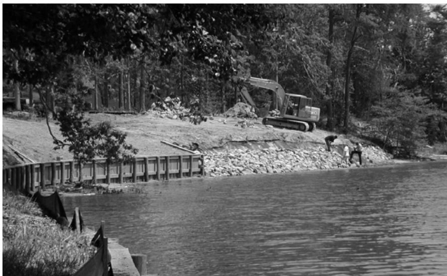
Figure 3. Piecemeal installation of erosion control structures by individual property owners results in cumulative impacts on living resources, such as tidal wetlands, important fisheries and riparian buffers.
